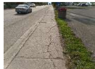
Sidewalk Cracking – Stuart Drive W
