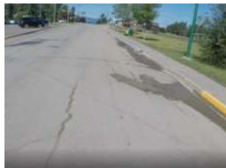
Inadequate Drainage – Stuart Drive E Near Curling Rink
