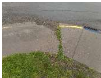
Tripping Hazards – Stuart Drive E
