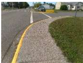
Sidewalk scaling – Douglas Avenue
