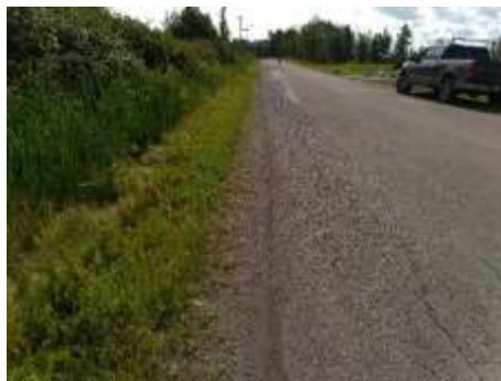
Ditch Vegetation and Ponding Water – Stones Bay Rd near Golf Course
