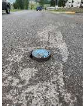
Protruding Valve Box and Loss of Surrounding Material – Stuart Drive E and Eagle Court
