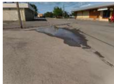
Surface Low Spot - Mason Street –
