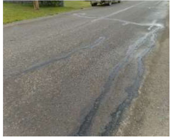
Level 3 crack seal condition
